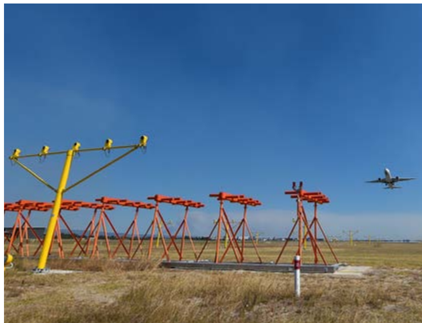
Figure 6-10 High Intensity Approach Light at Perth Airport Source: Perth Airport
